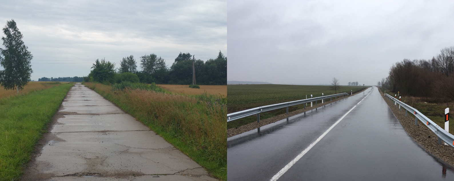
The local road, which was sometimes used by military traffic, had become cracked and damaged due to settlement of the underlying weak clay soils. Photos of the road before and after reconstruction.
