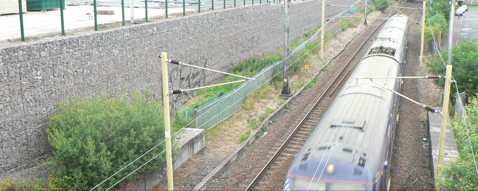
The new perimeter retaining wall forms an attractive boundary alongside the Glasgow-Edinburgh railway line.
